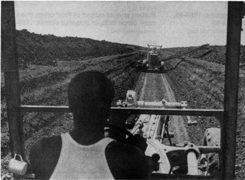
Construction of a canal in Rahad, Sudan. One of Sudan's priorities to accelerate development is to make existing water resources more readily available for domestic, agricultural, and industrial use.
