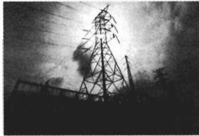
An aluminum tower, holding aluminum electrical transmission cable aloft.
