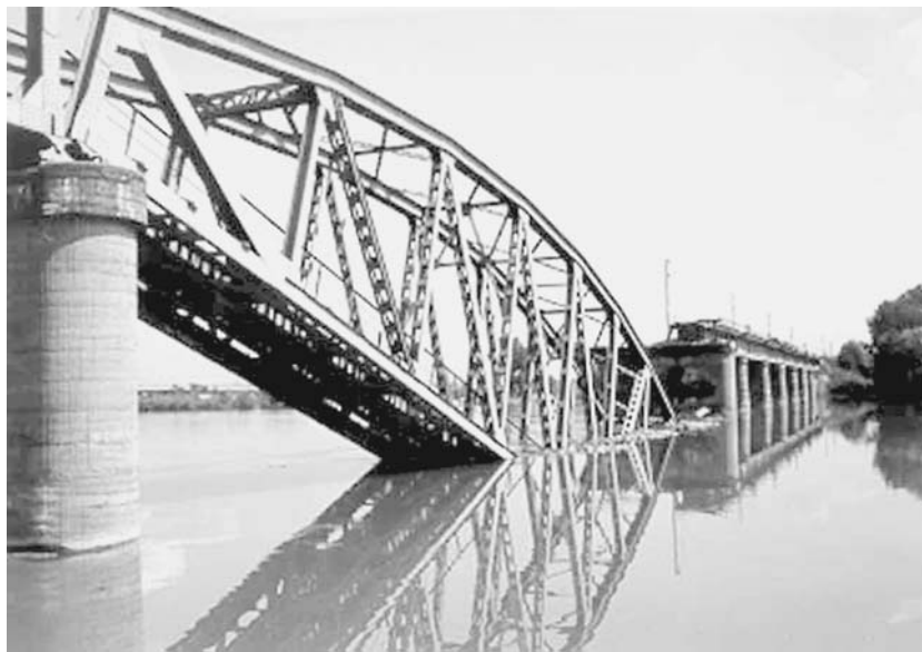
The Ostruznica railway bridge in Belgrade, destroyed by NATO bombing in May 1999.
