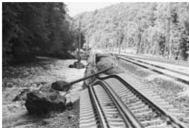
Floods of August 2002, which destroyed roads, bridges, and railways across Germany, added to the already severe transport deficit caused by a decade of austerity against planned investments. This stretch is between Dresden and Tharandt.
