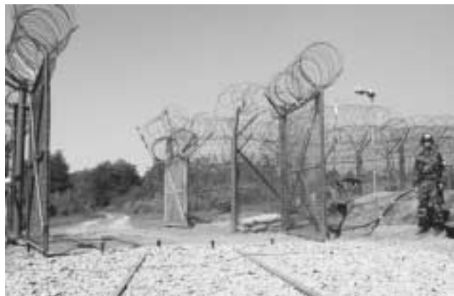
Rail corridor construction opens the two Koreas’ long-forbidden border. Gates are open at the DMZ after 50 years—to allow the construction of new rail lines up the whole peninsula, the Eastern end of the “New Iron Silk Road” across Eurasia. This is a major objective of LaRouche’s New Bretton Woods monetary reform.
