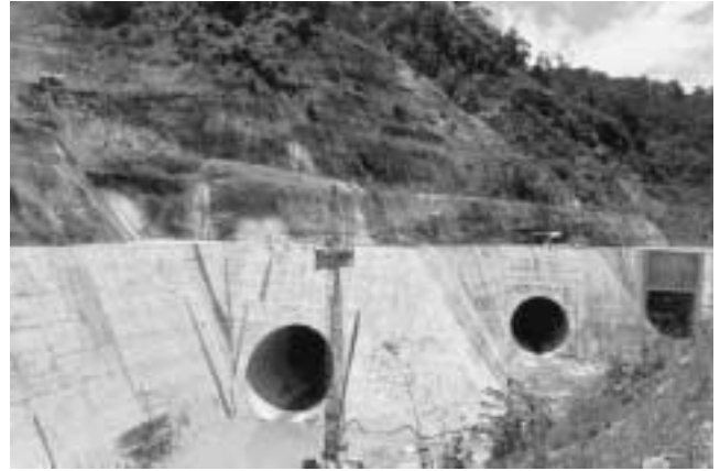
Diversion tunnels have already been drilled in preparation for the dam construction.
