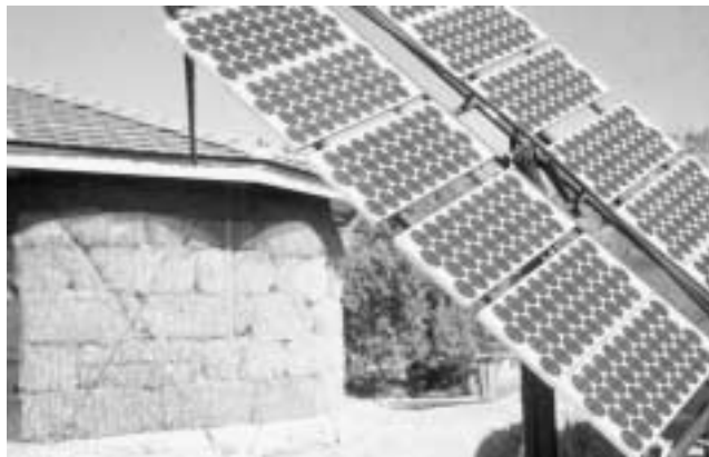
Solar power as infrastructure.
