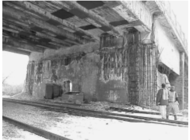
The aging Rockefeller Road Bridge, Cleveland, Ohio, is one of many decaying bridges over the rail corridor.
