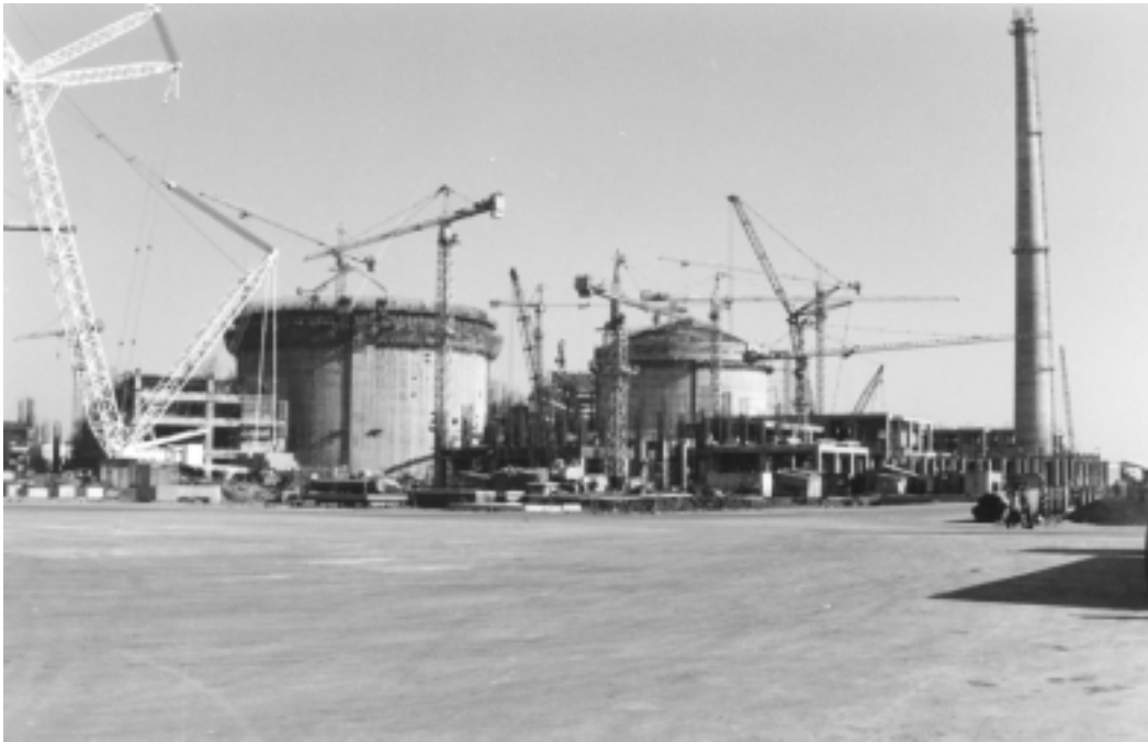
The first of India's pressurized heavy water reactors, a 540-MW unit, located at Tarapur. A second unit will be commissioned there this year.
