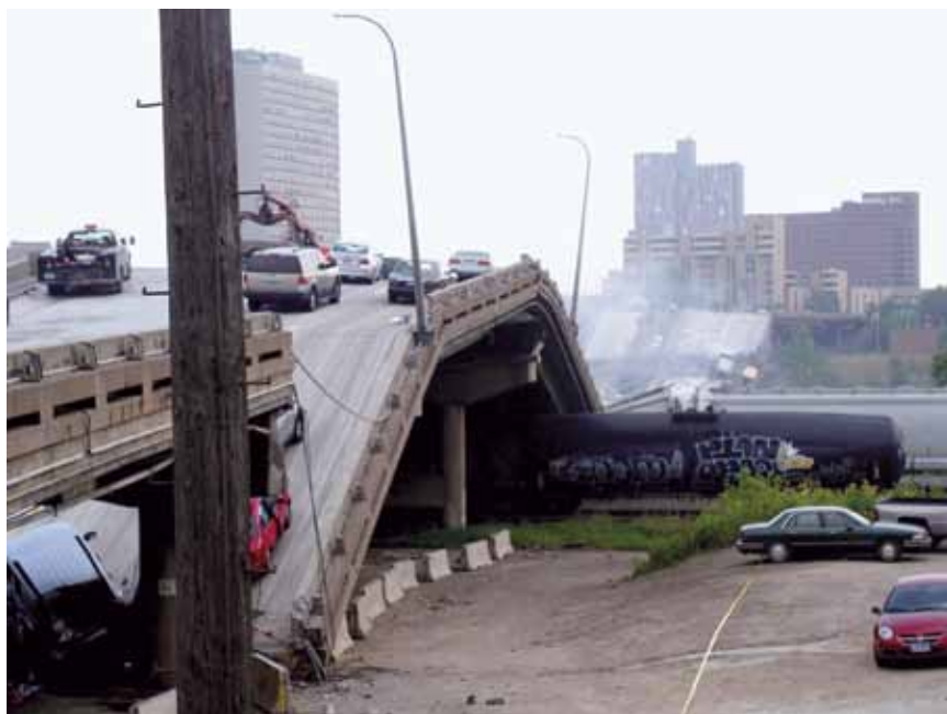
The I-35 bridge collapsed into the Mississippi River in Minneapolis, Minnesota on Aug. 1, 2007.
