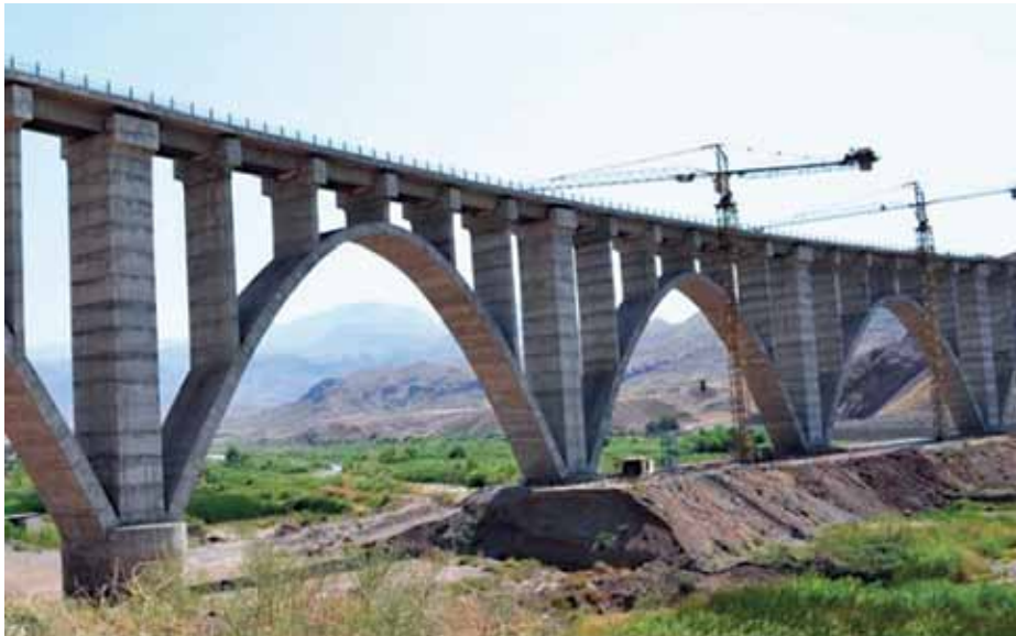
A railway viaduct on the Rasht-Astara section of the INSTC nears completion.
