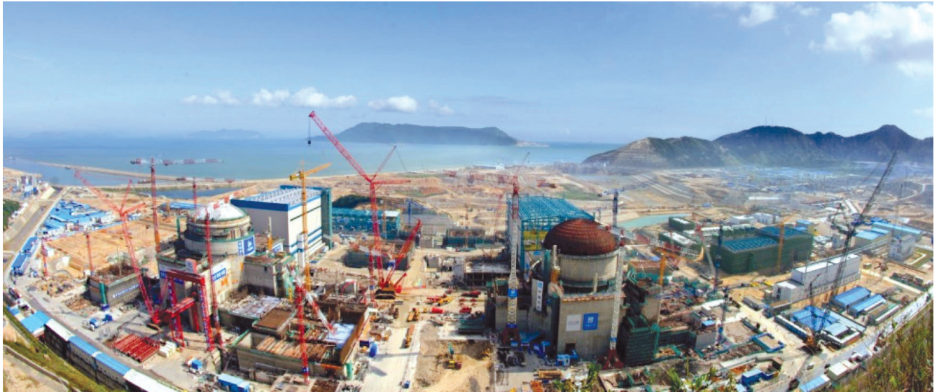
The two-unit Taishan nuclear power project, using advanced, third-generation nuclear power technology, under construction in Chixzhen, Taishan, Guangdong province, China. It is a China-foreign joint project with large participation by Areva and Electricité de France. The bulk of French electricity production is nuclear powered. France exports electricity to Germany, which is stupidly shutting down all its nuclear plants by 2022.
