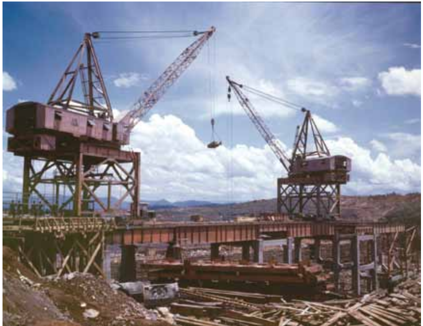
LoC Construction work at the TVA’s Douglas Hydroelectric Power Dam, on the French Broad River in Tennessee, June 1942.
