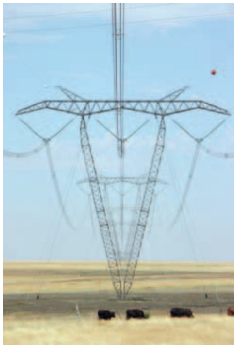
Eighty-five percent of South Africans have access to electricity. Here, an electrical power transmission pylon.
