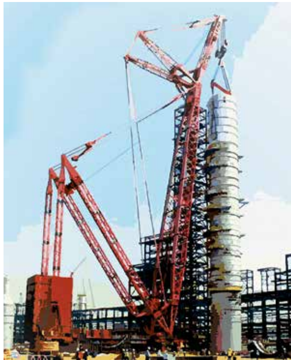
The world's largest distillation column being erected at the Dangote refinery in Lekki, Nigeria, just east of Lagos.
