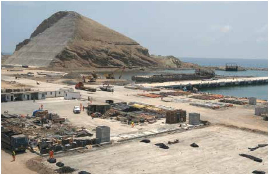
Chancay Port on the Pacific coast of Peru, a “megaproject” being developed with China, pictured here in June 2024, which will be inaugurated by the presidents of China and Peru on November 14, 2024.
