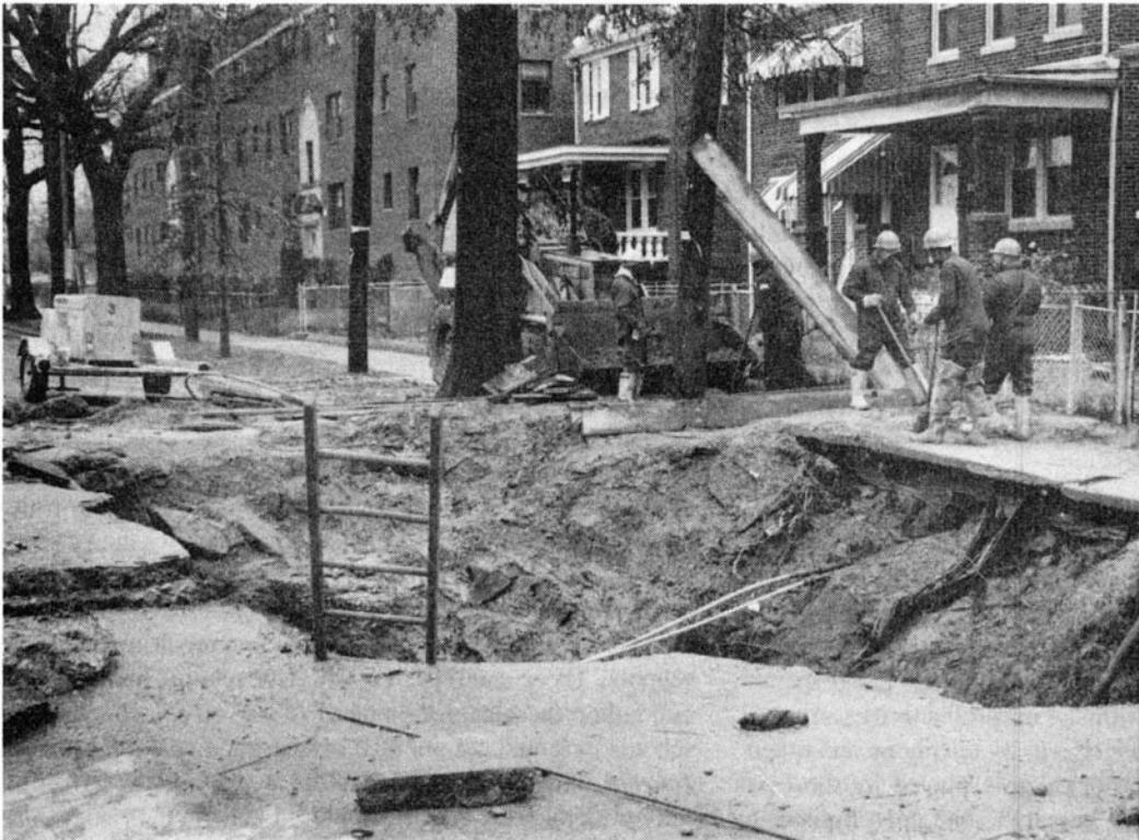
Workers repair a water main break in Washington, D.C. in November 1993. The decay of urban infrastructure long predates the January cold snap, being the result of 30 years of incompetent economics.
