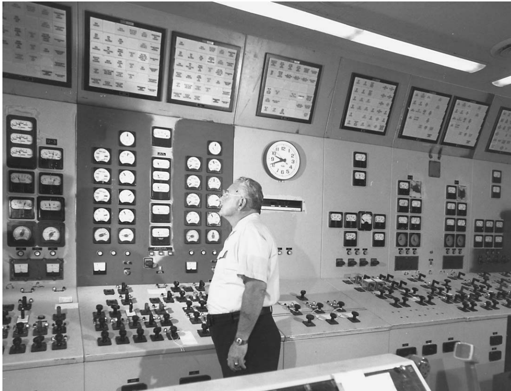
The control room of the Shasta Powerplant near Redding, in California's Central Valley. In Los Angeles, the Department of Water and Power is now laying off 2,000 engineers, technicians, and managerial workers—slashing the skilled workforce on which the nation's future development depends.
