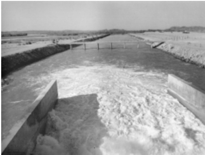
The 80-mile All-American Canal, looking from the overflow section of the Imperial Dam on the Colorado River. These waterworks were built during FDR's New Deal. The Canal, completed in 1940, began carrying water in 1942, to eventually irrigate some 500,000 acres in the Imperial Valley, through a system of 2,900 miles of laterals. Ditches carry off surplus water to the Alamo River. The Imperial Dam, completed in 1938, was the second on the Colorado, after the Hoover Dam. The Canal is among water and power installations run by the Imperial Irrigation District, set up in 1911 to administer power and water to a service area today covering 6,471 square miles in the Valley.
