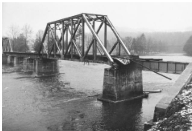
The failure to maintain infrastructure is a form of looting the physical economy which can be disguised—up to a point.
